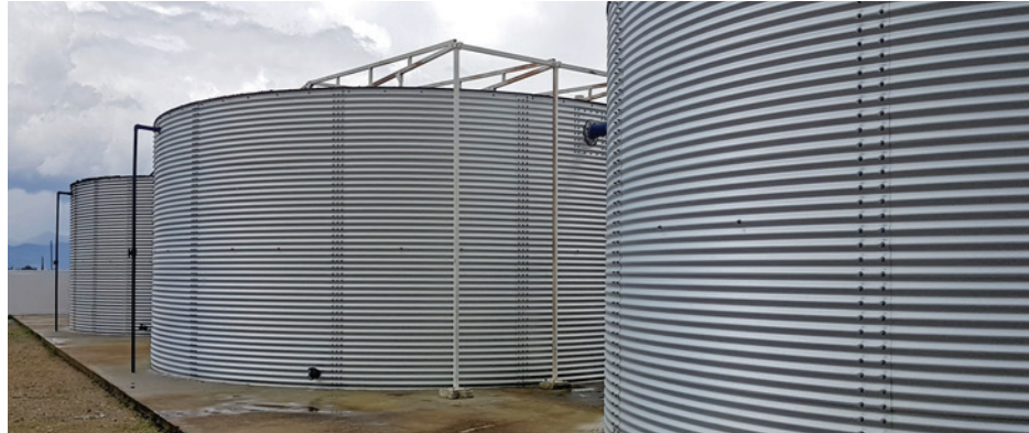
Water Treatment Plant, Del Toro
